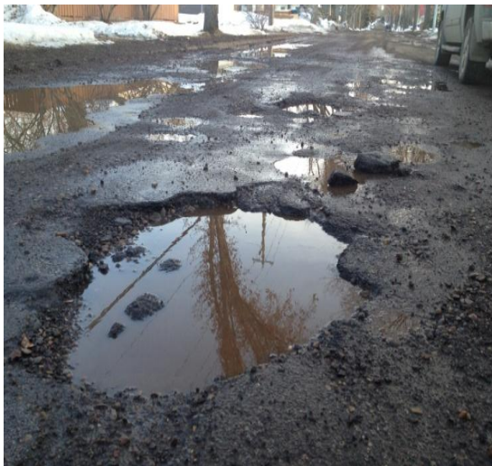
Fig1:-Potholes on Road
