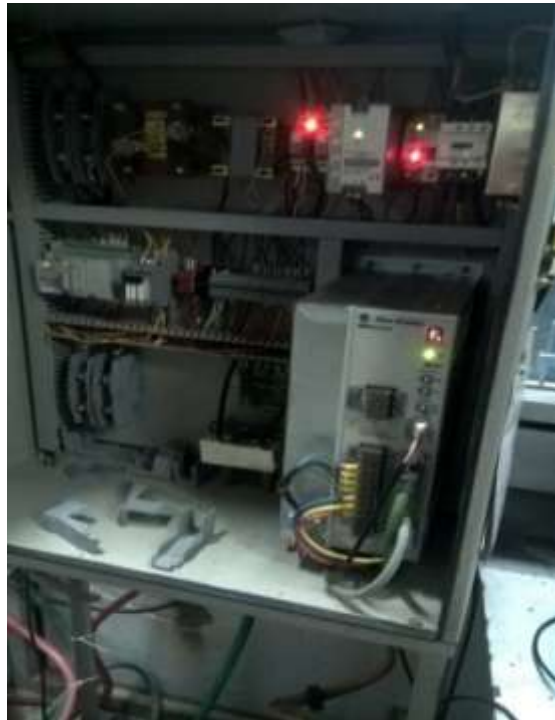
Fig 2. The Welding System Control Panel
