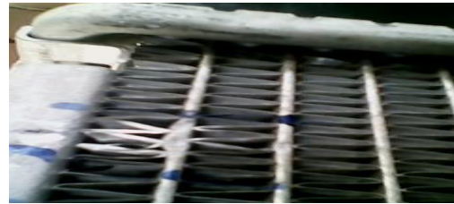
Figure 3: Defected Dent Tube
