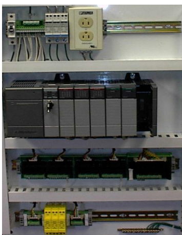
Fig 4: Control panel with PLC (grey elements in the center). The unit consists of separate elements, from left to right; power supply, controller, relay units for in- and output.
