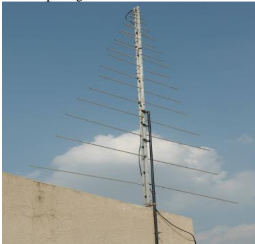
Fig. 1. Photograph of installed LPDA
