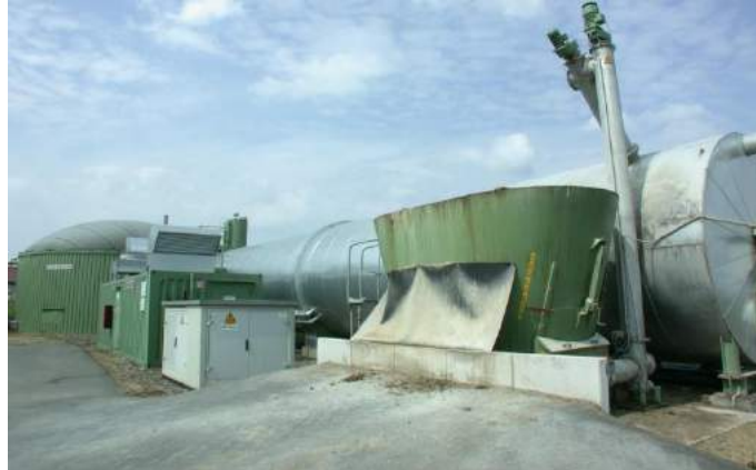
Fig.1 farmyard anaerobic digester converts waste plant material and manure from livestock into biogas fuel.
