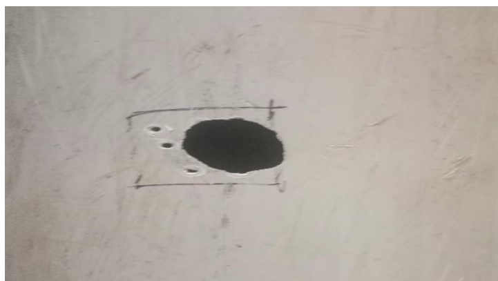
Fig 3.3: Crack in the pipe
