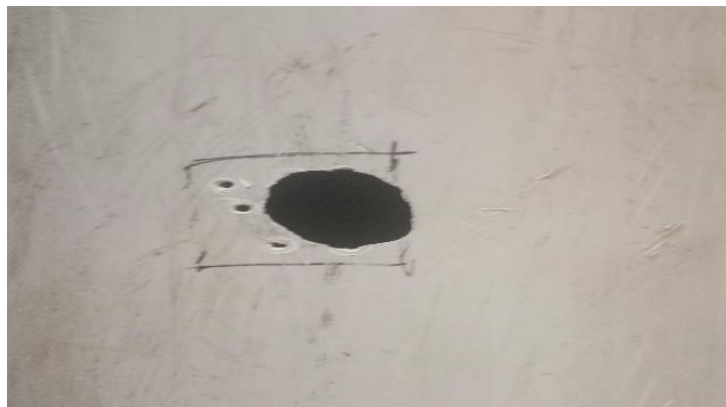
Fig 3.3: Crack in the pipe
