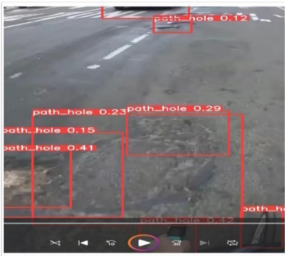
Figure 6.6: Detected Pothole using Videos
