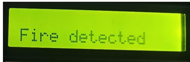
Fig: 4 LCD Displaying Fire Detected
